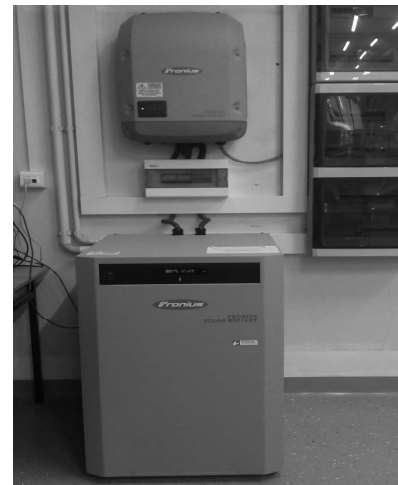
Fig. 2. Fronius Symo Hybrid 5.0-3-S S24 together with Fronius Solar Battery in the laboratory of UTP in Bydgoszcz
